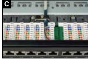
Check and ensure each wire in correct slot.
